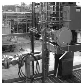
INDUSTRIAL PLANT USINE PLANTA INDUSTRIAL
